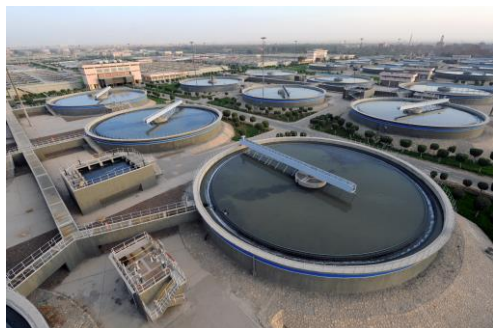
The Gabal El Asfar wastewater treatment plant in Cairo - Copyright : Thomas Goisque
