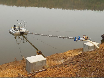
Floating barge for pumping water from Lake Bakro
