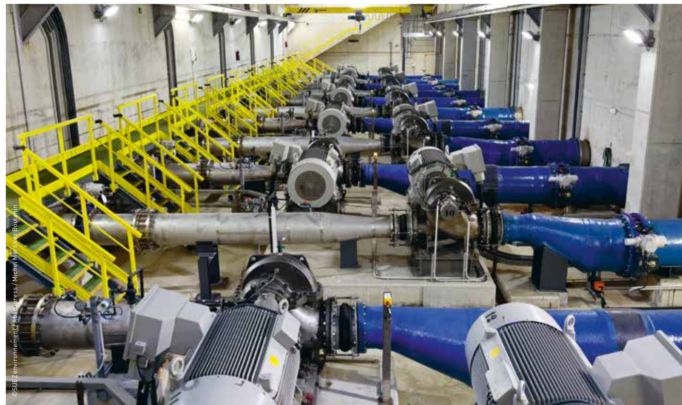
Intermediate pumping between the first and second filtration step
