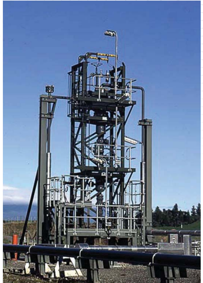
Shell Mangahewa CYCLONIXX® Wellhead Desander Package Location: New Zealand
