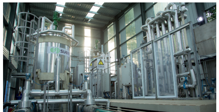
full-scale demonstration unit in Handan, China
