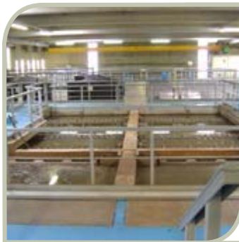
Waste water treatment plant (Biarritz, France)
